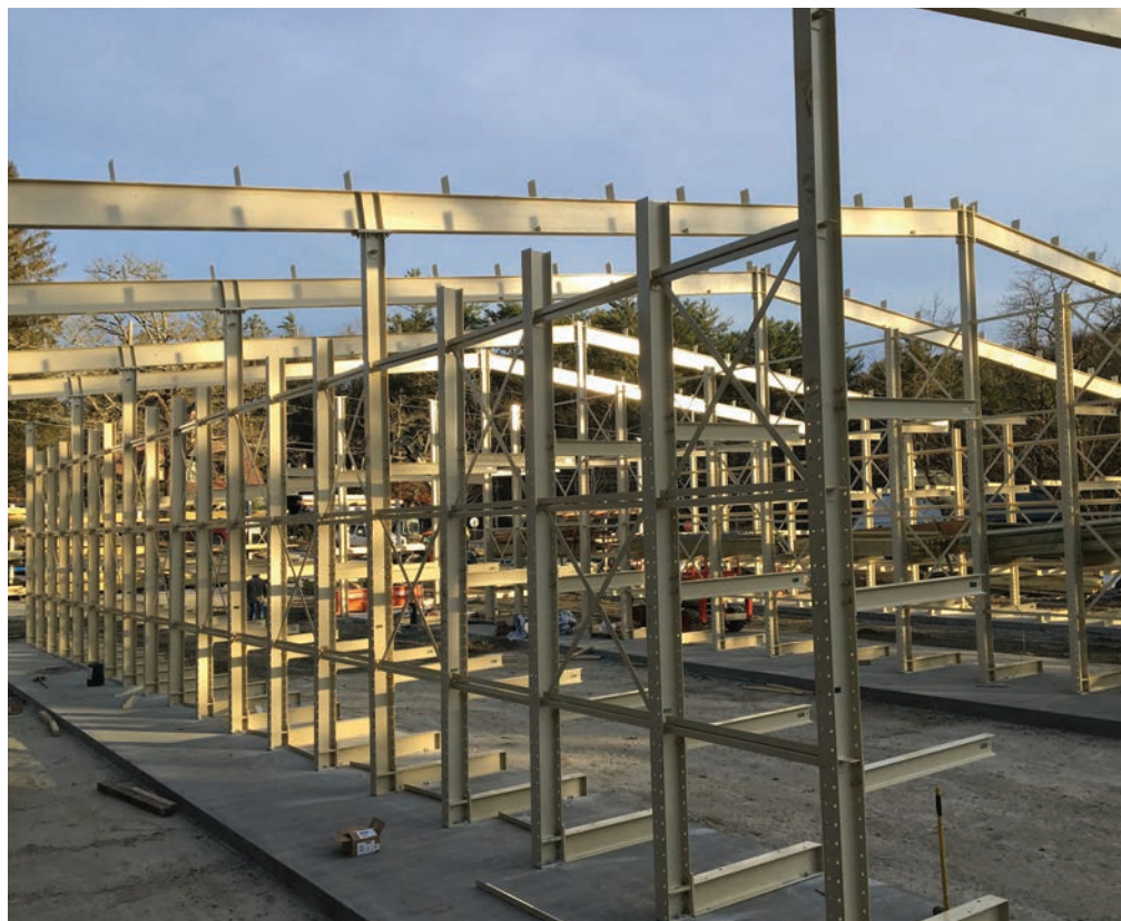
RACK-SUPPORTED structure designer/builder was able to offer sole-source responsibility, resulting in a seamless interface between engineering and marketing.
